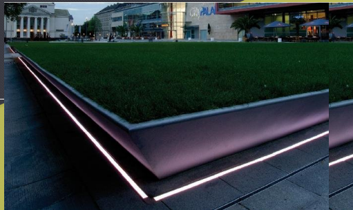
Intra LED lines mounted flush with pavement
